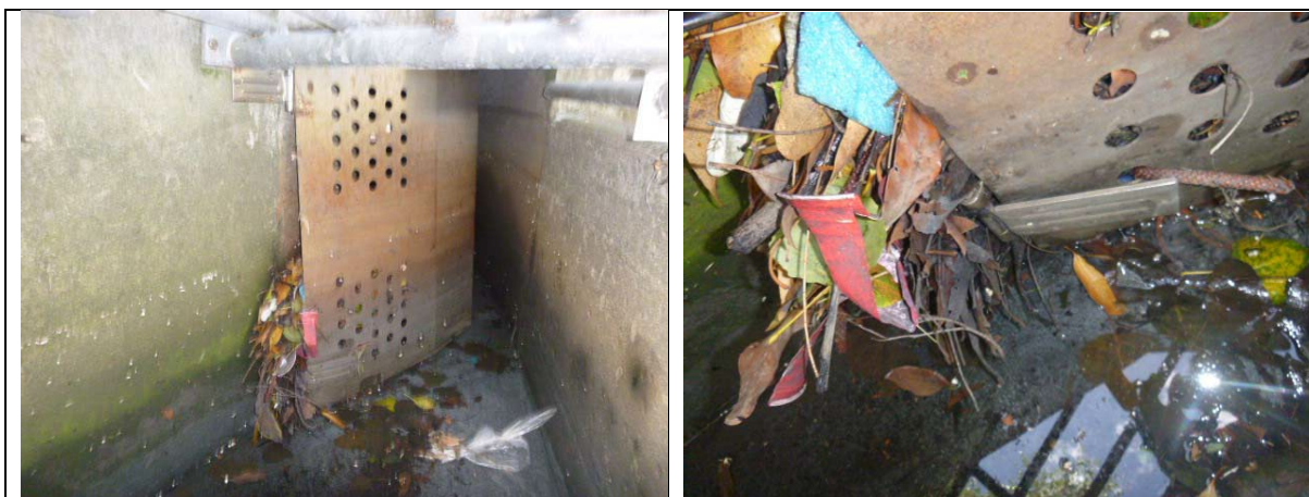
The floatables flap was jammed open due to a broken hinge and pollution trapped in it stopping it closing.
