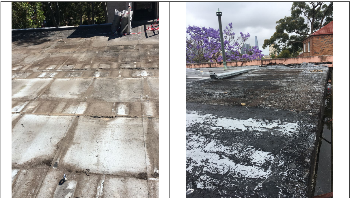
Examples of failed waterproofing on flat roofs
