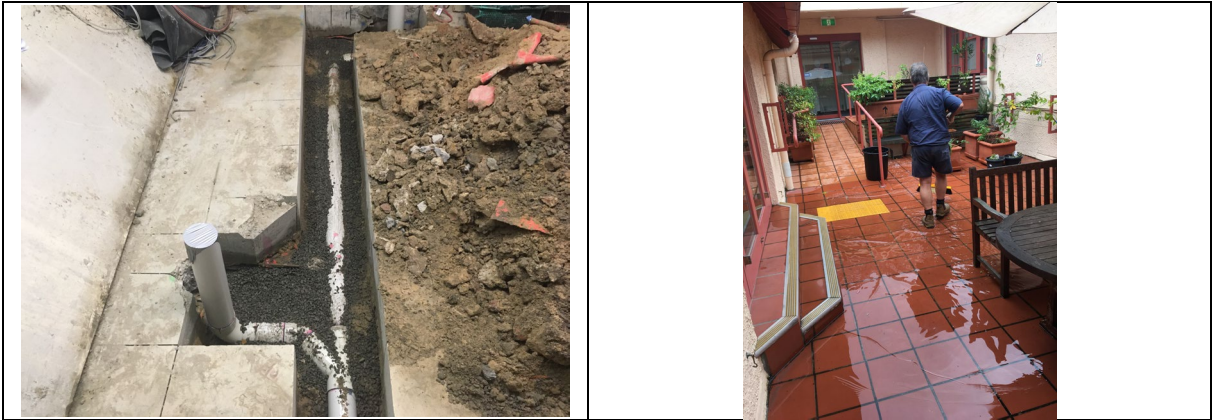
Examples of failed sewer and stormwater pipes
