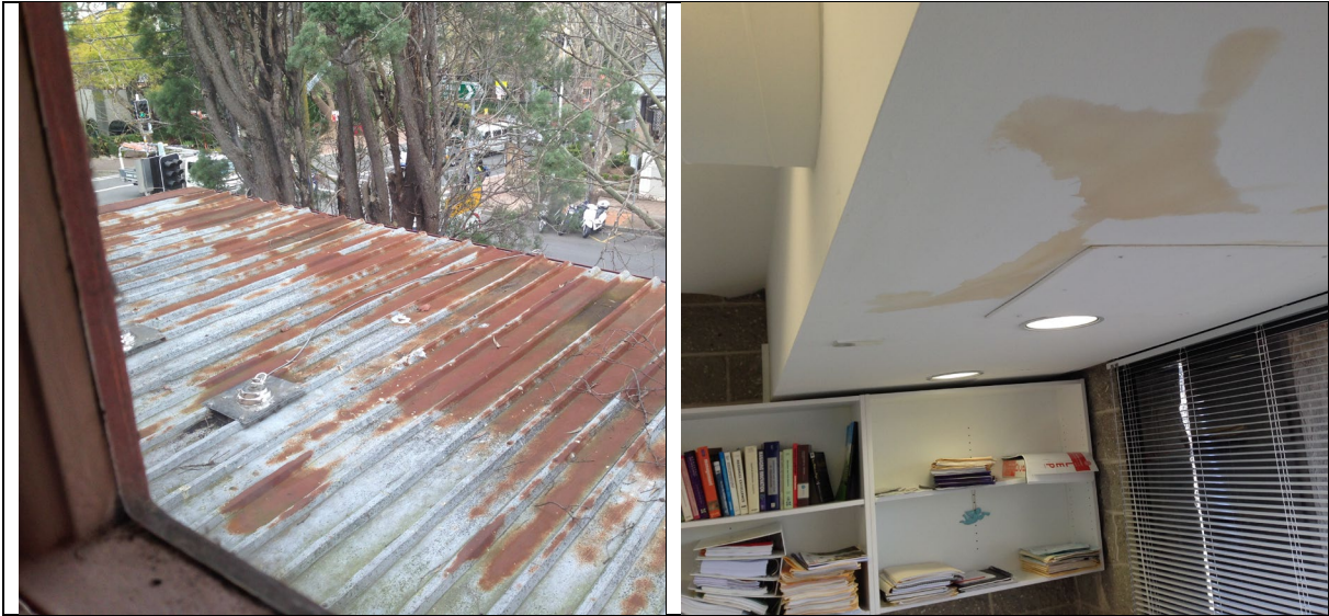
Examples of failed and failing Property Assets in the North Sydney LGA
