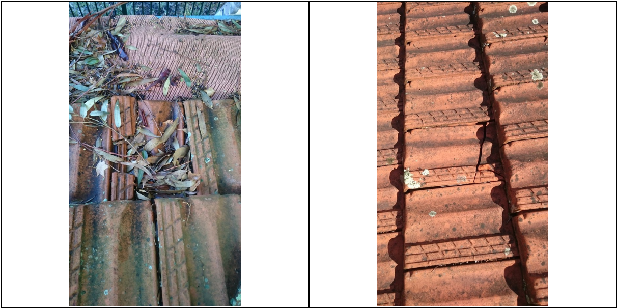
Examples of cracked roof tile Assets in the North Sydney LGA
