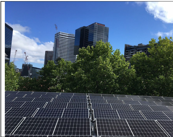
Solar Panels have been rolled out across a number of Councils Community and operational buildings over the last 5 years as part of an ongoing program. North Sydney Council Chambers Wyllie Wing roof
