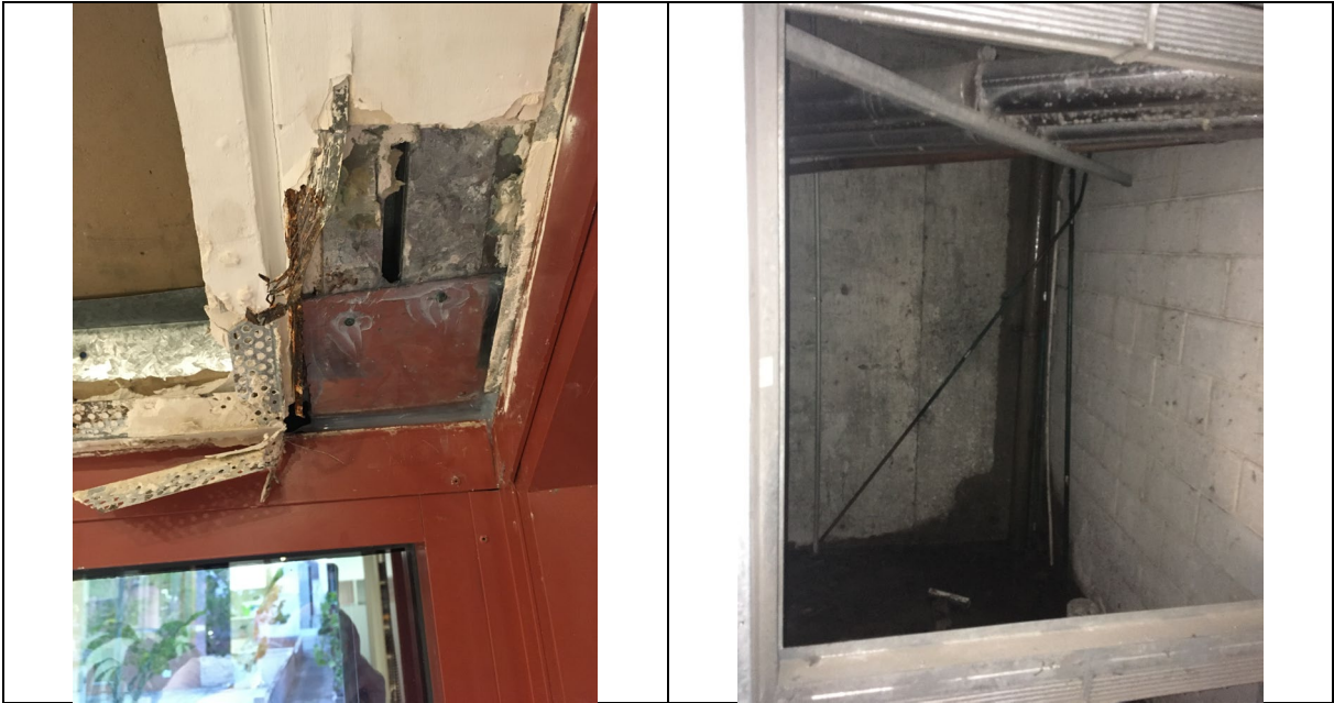
Examples of failed and failing Property Assets in the North Sydney LGA
