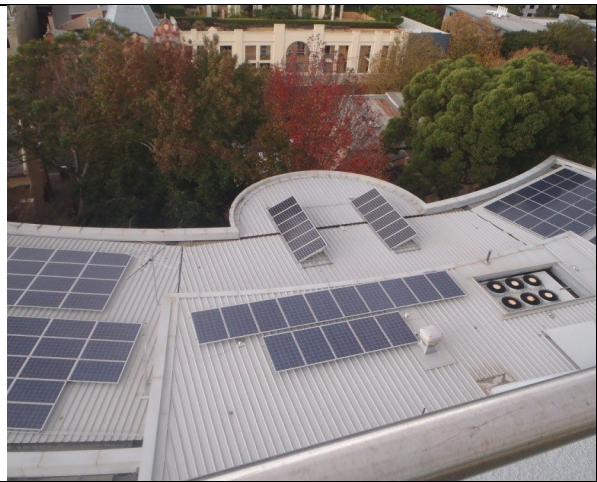
Solar Panels have been rolled out across a number of Councils Community and operational buildings over the last 5 years as part of an ongoing program. Stanton Library
