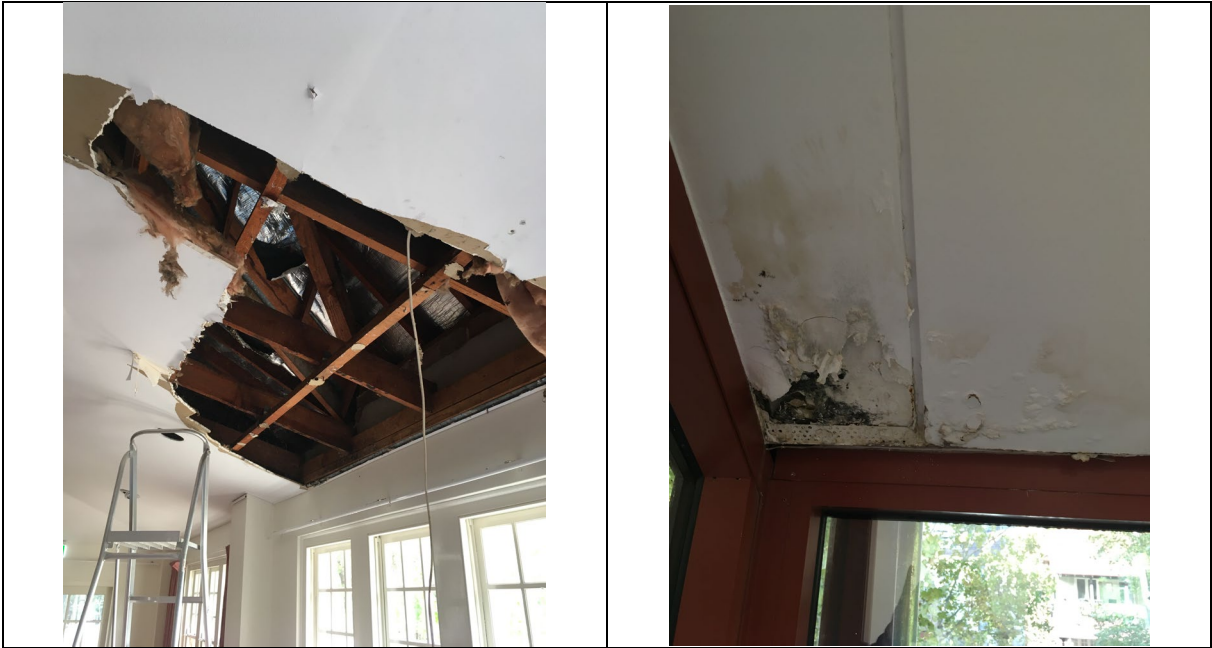
Examples of leaky roof Property Assets in the North Sydney LGA
