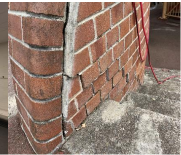
Poor/ Very poor:
