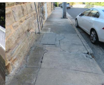
Poor/ Very poor:
