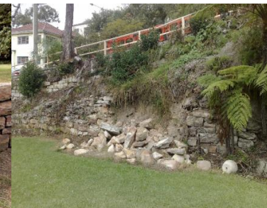
Poor/ Very poor:
