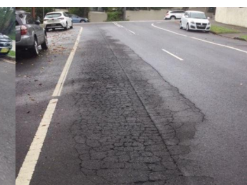
Poor/ Very poor:
